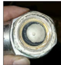
Rubber Degrading – Leaking Likely
